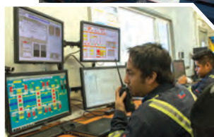
Power plant control room
